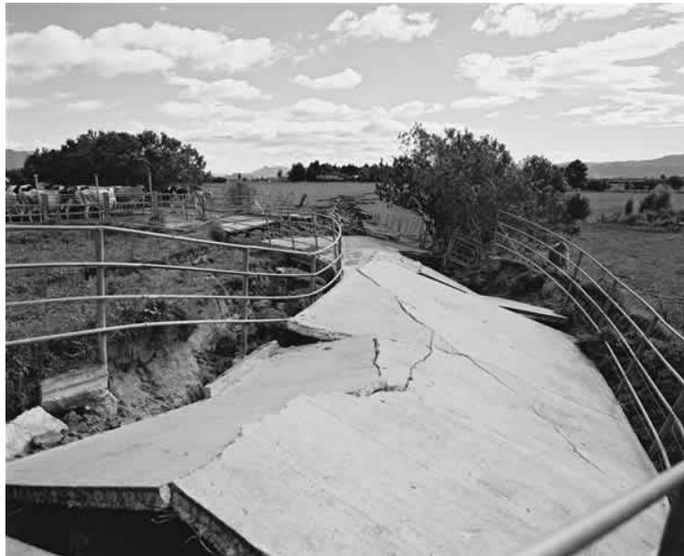
Road Damage Caused by an Earthquake
